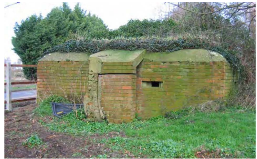
(Above: The Meadow Bridge pillbox a few years ago. It's now almost entirely hidden by vegetation)
